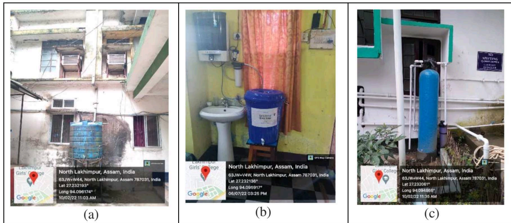
Figure 5: (a) Rainwater Harvesting (b) Collection of waste water from RO filter (c) Groundwater extraction
